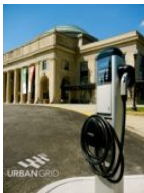
Chargers installed at the Science Museum of VA (Credit: Urban Grid Solar)
