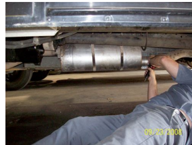
Figure 3: Muffler after DOC installation
