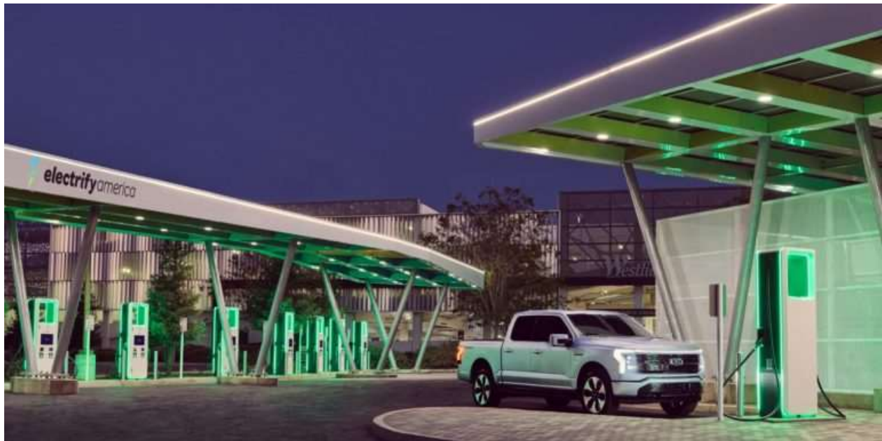
Figure 62. Electrify America DCFC Charging Plaza in Santa Clara, CA
