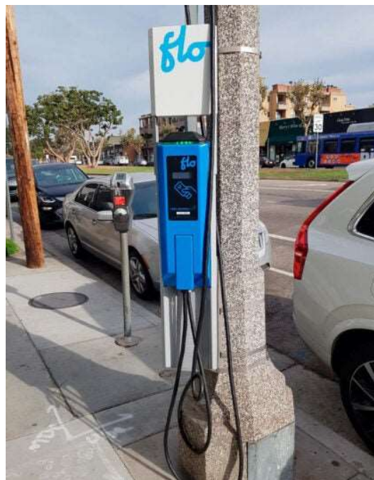
Figure 67. Streetlight EV charger in Tacoma, WA Credit: Tacoma Public Utilities
