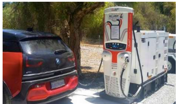
Figure 72. Fixed Diesel Generator Powering an EV Charger
